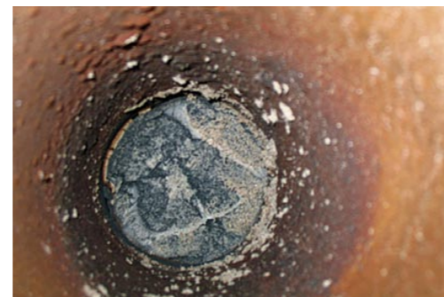
After the test (pipeline obstructed by the intumescent material)
