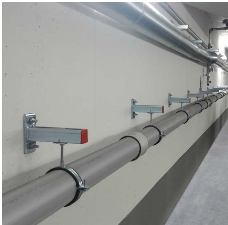
Considerable bracketry and fixing expenditure on a plastic pipeline
