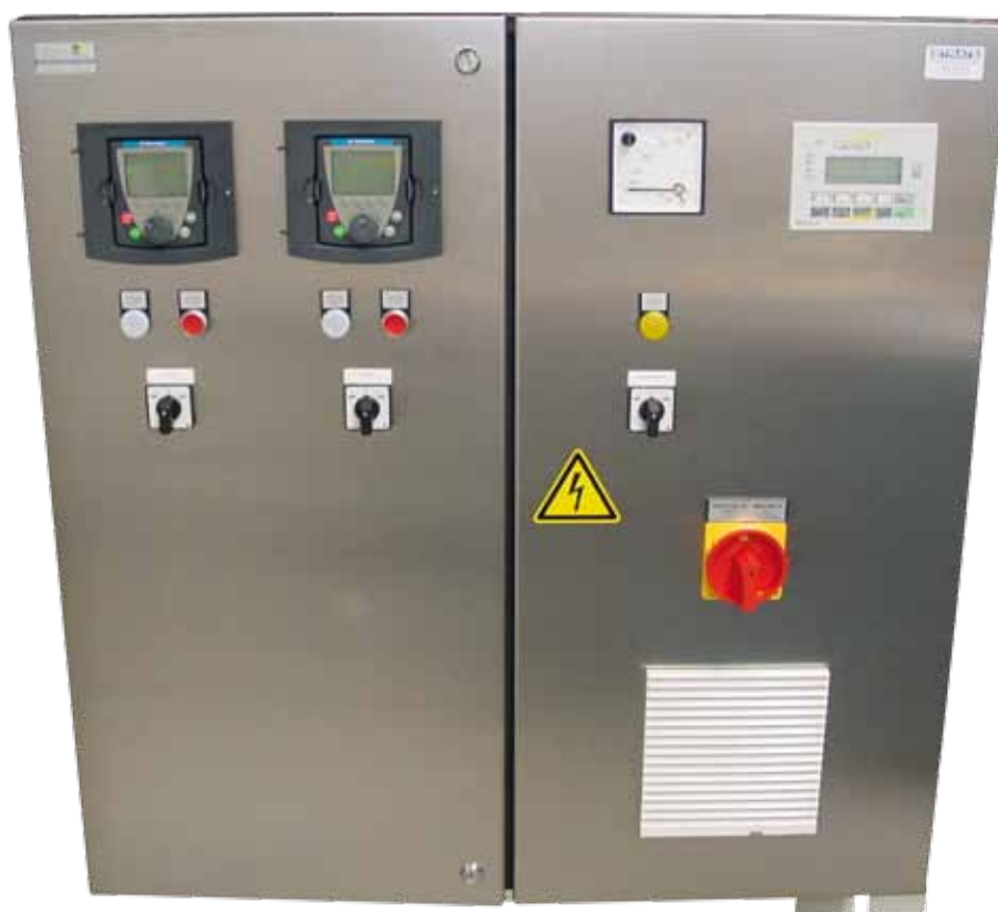
ED control cabinet
